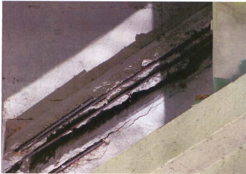
SPALL W/EXP REBAR ON DIAPHRAGM BTWN BEAMS C & D JOINT @ PIER-2
